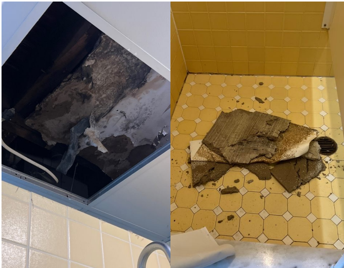
Photos of some of the damage caused by the plumbing issues over winter break. Photo credit: Cate Cheng
